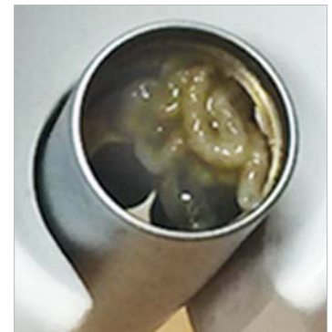
Figure 1a. Slime worm released during handpiece flushing. Taken from working dental office by service representative.
